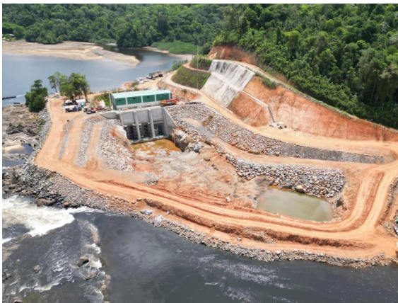
Cafesoca hydroelectric plant
